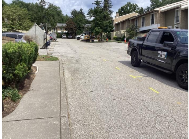
Asphalt pavement overview with cracks
