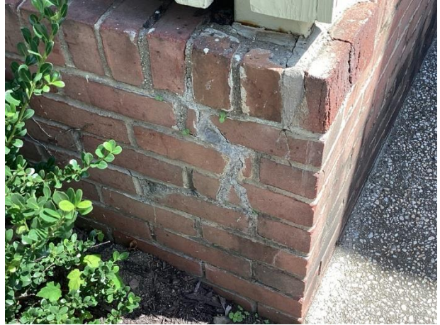
Cracks and repairs
