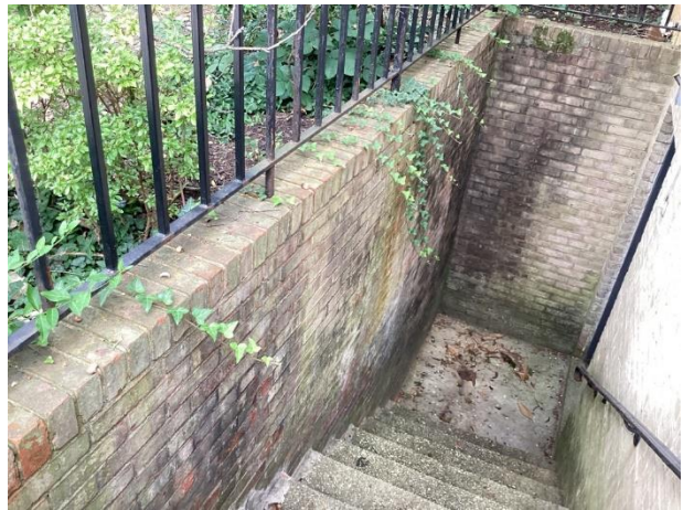
Masonry retaining wall overview with organic growth
