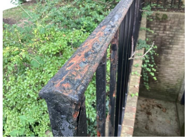
Rust and finish deterioration
