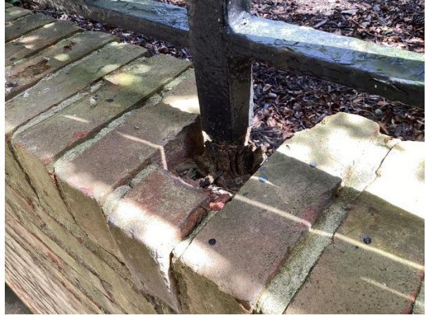
Masonry deterioration at railing attachment
