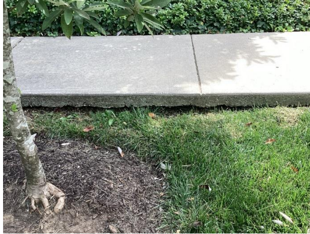
Soil undermining at sidewalk
