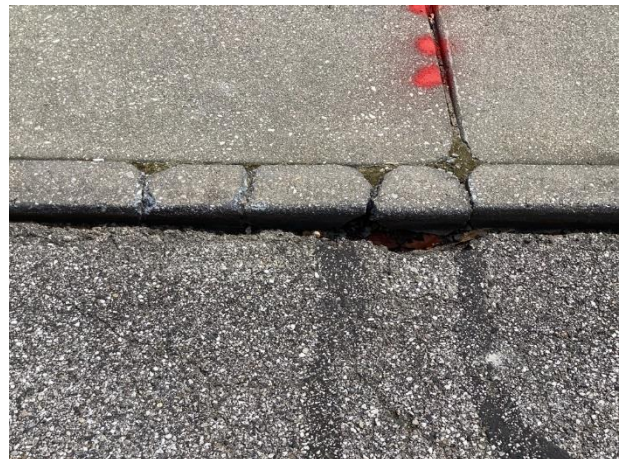
Concrete cracks and organic growth
