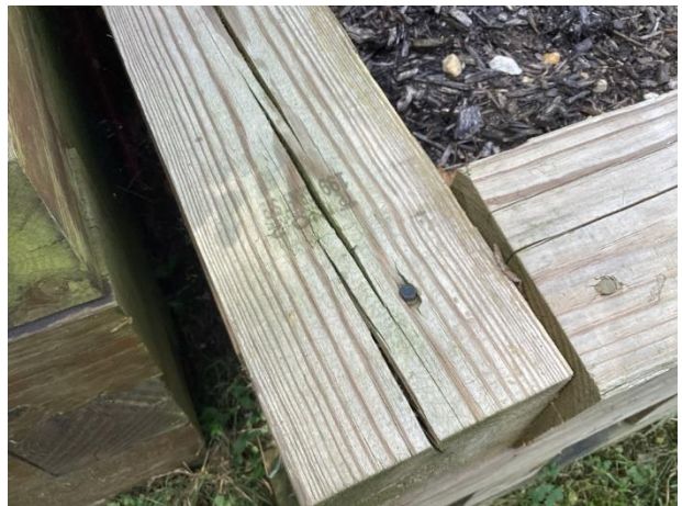
Repairs and wood deterioration
